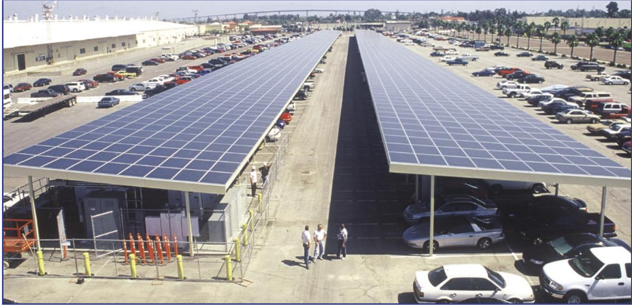
The solar photovoltaic array at Naval Air Station North Island, the world's largest covered parking solar installation. (Photo Credit: Naval Base Coronado)
