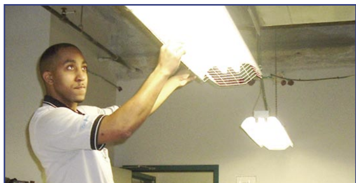
CHCC Plant Services staff member Edmond Logan installs a new, more efficient lighting system. (Photo Credit: Children’s Hospital Central California)
