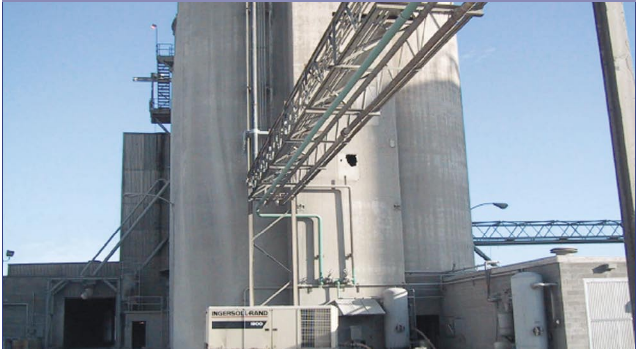
New air piping at California Portland Cement Company's cement factory helps to reduce the energy use of the compressed air system. (Photo Credit: California Portland Cement Company 25 )
