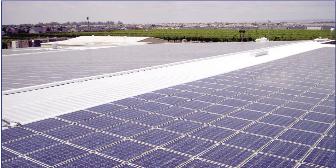
Pat Ricchiuti, owner of P-R Farms, completed installation of this massive solar array in July 2005. The system consists of 7,730 panels, covering 98,100 square feet. It reduces California's global warming pollution by over 1 million pounds per year. (Photo Credit: PowerLight)
