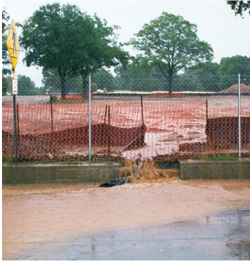
Figure 6. Construction site with inadequate sedimentation 95
