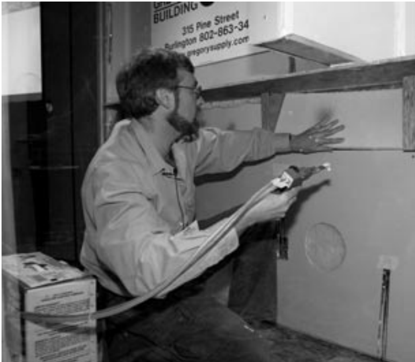
Foam panel insulation is sealed around the edges with spray foam. New building materials can greatly improve the efficiency of old and new buildings alike.
